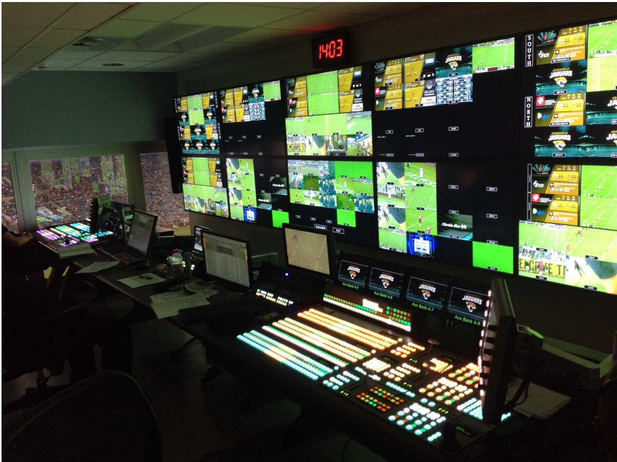
The new Jacksonville Jaguars control room features two Vision Production Switchers, a Carbonite frame acting as an image processor for the 8K board, XPression Studio graphics engines, as well as the Inception Social system.
