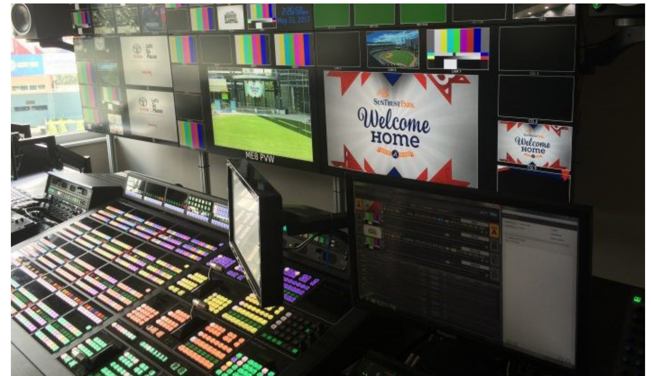
An Acuity Production Switcher anchors the state-of-the-art Production Control Room.
